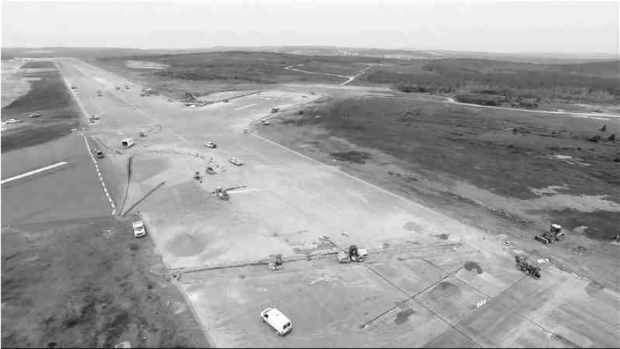
Reconstruction at the intersection of the primary and secondary runways at YYT got underway in early July, imposing significant operational restrictions. When bad weather struck, chaos resulted. But the project means better days are ahead. (PHOTO: St. John’s International Airport Authority)
